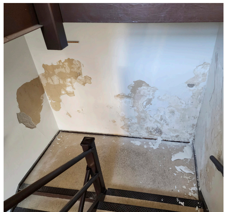
Plaster peels away from the wall at IDOT's Ash Street facility in Springfield.
