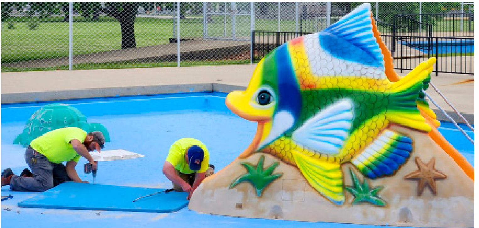
Members of Local 2050 make repairs to Springfield's public pool before summer begins.
